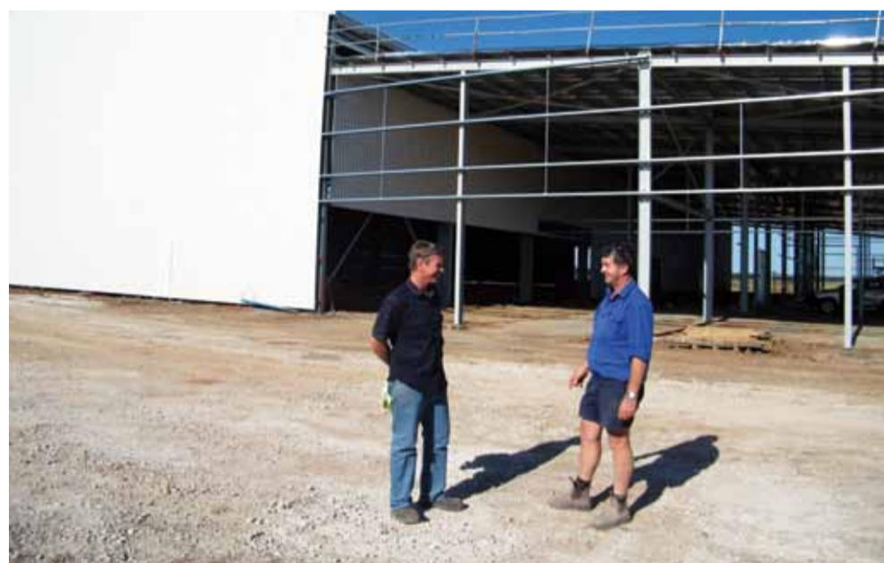
Above: Gin manager Chris Veness with Roger Commins inspect the construction of the new cotton gin near Winton.
